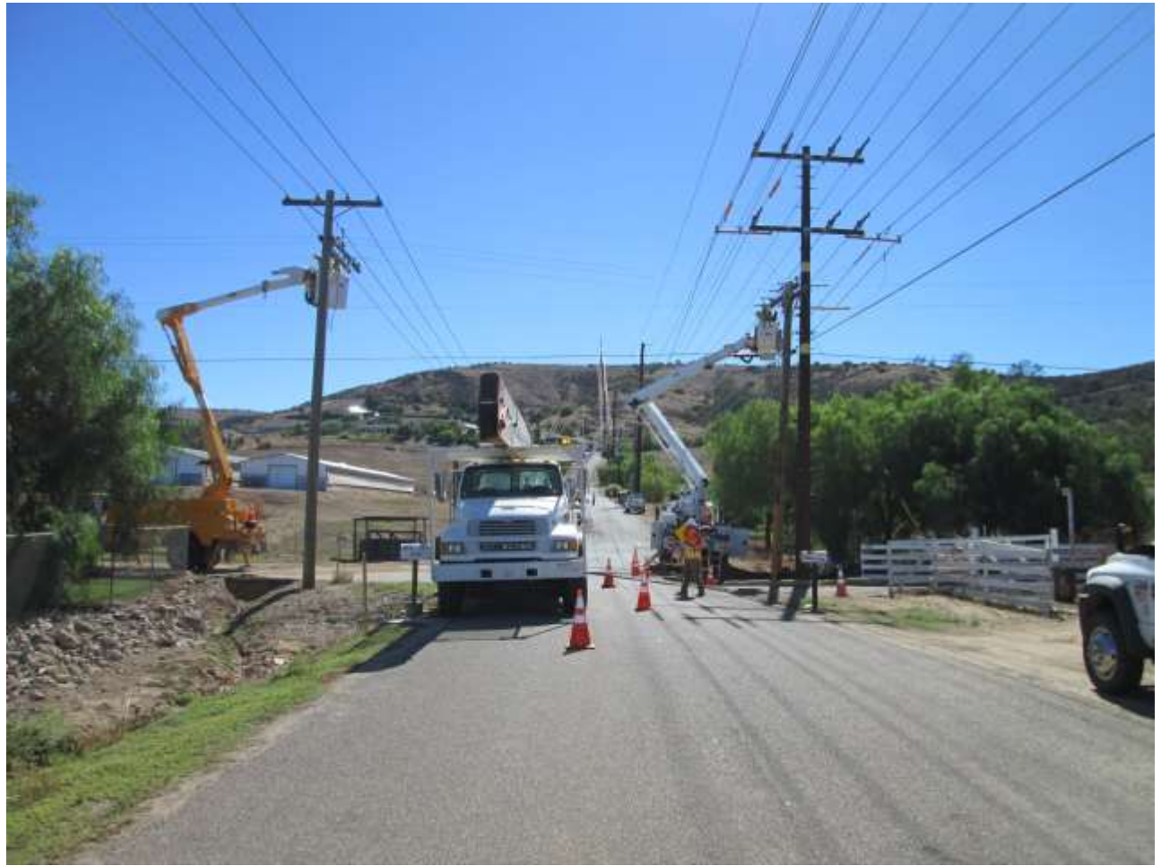
Photo 7: Crews were observed wrecking-out poles and replacing a 12kV conductor line while implementing traffic control measures (APM TRA-1) and fire prevention measures (APM-HAZ-2).
