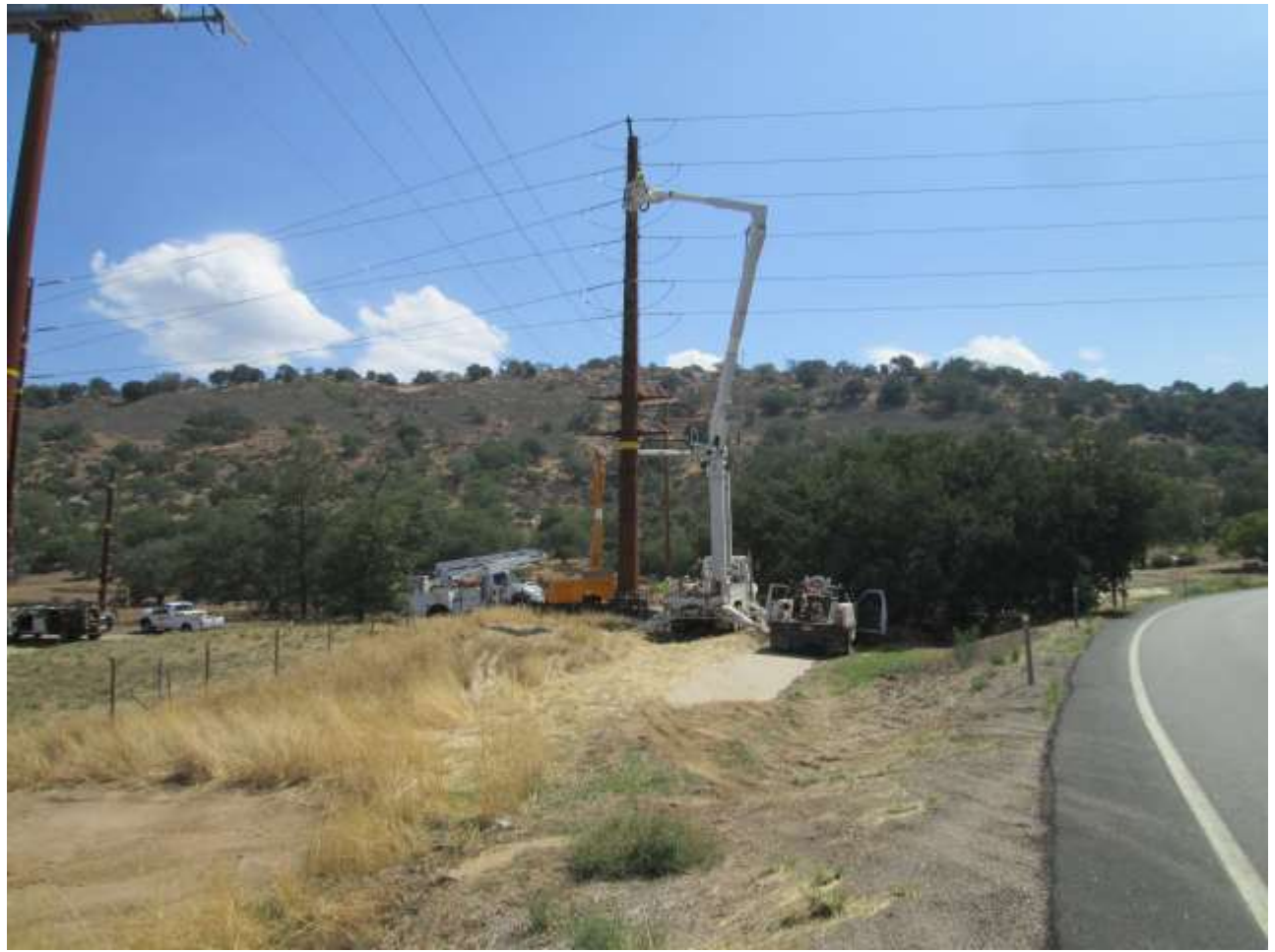
Photo 6: Crews were observed conducting overhead line work inspections, such as x-raying dead-end poles.
