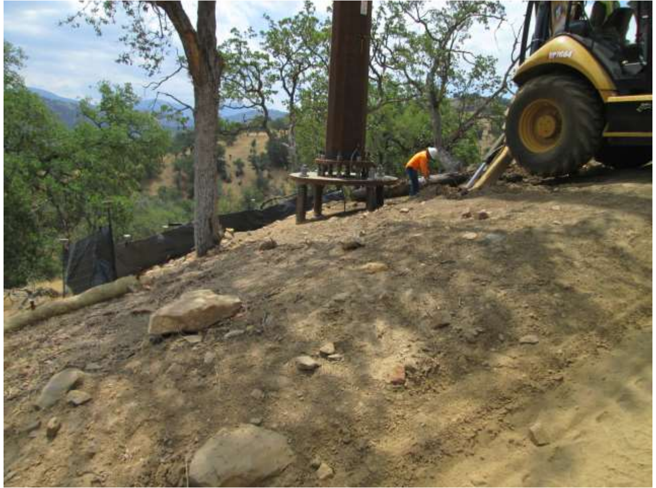
Photo 3: Erosion control BMPs (straw wattles and silt fencing) were observed intact during wooden pole butt excavation and removal at Location 139.
