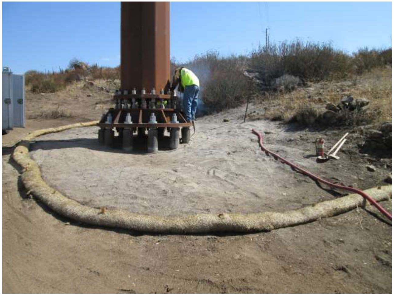
Photo 5: Crews were observed welding micropile foundation nuts. Preventative fire measures including carrying fire equipment (fire extinguisher, shovel, and pulaski), performing work in cleared spaces, and having a water tender with hose mobilized adjacent to the work space were observed during welding activities in accordance with the Project Fire Plan.
