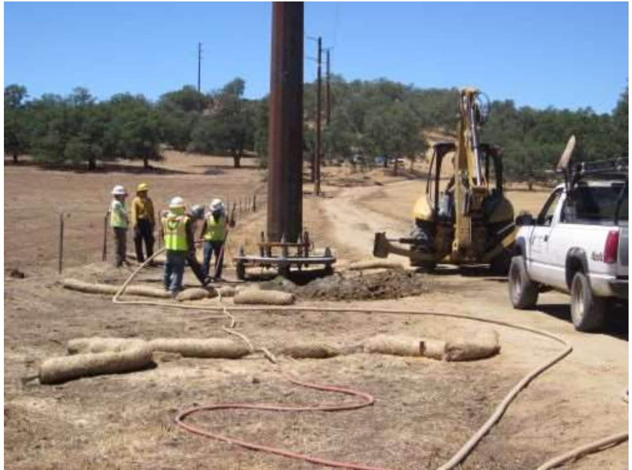
Photo 1: A biological monitor and aquatic resources monitor observe wooden pole butt excavation removal at Location 146 in accordance with MM BIO-2 and APM HYD-1.
