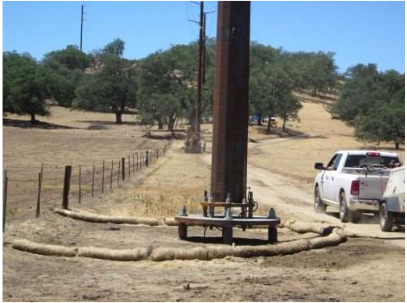
Photo 2: After wooden pole butt excavation occurred at Location 146, erosion control BMPs (straw wattles) were observed replaced in accordance with the project SWPPP.
